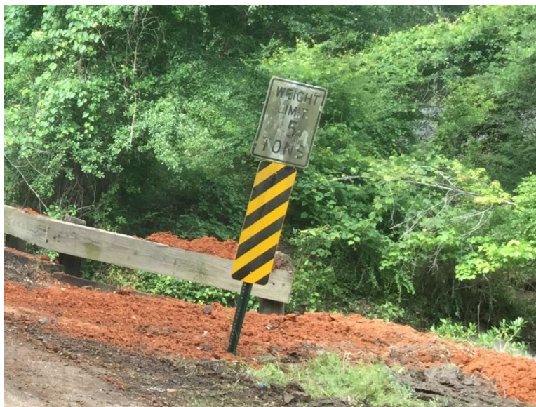
Figure 3-13: Illegible weight limit sign
